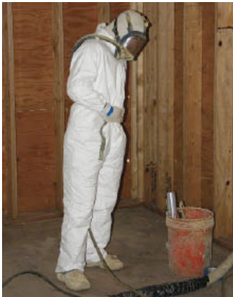
Figure 5. A supplied-air respirator is a must when spraying foam. A layer of clear plastic wrap keeps the face shield clean for repeat use.
