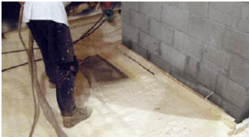
Figure 2. The foam can be walked on only minutes after spraying, permitting multiple layers without significant delay. The 2x4 at this chimney base will be removed after spraying to provide the code-required gap between the flue and the foam.
