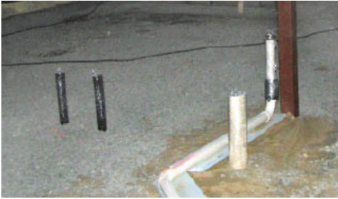
Figure 3. Cured foam sticks tenaciously to most surfaces. Plastic food wrap protects these plumbing stubs from the overspray.
