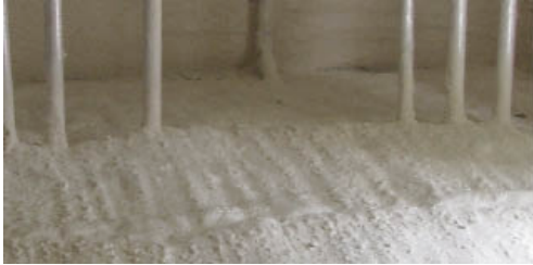
Figure 1. Plumbing penetrations can be tricky to plug with rigid foam board; SPF seals seamlessly around obstacles with a few passes of the spray gun.
