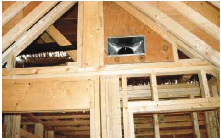
Figure 6. Here, a forced-air register is installed in a piece of 3/4-inch plywood where it penetrates the attic air barrier. The register boot is caulked to the plywood.
