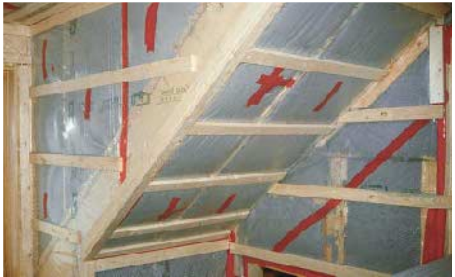
Figure 3. When the budget allows, 2x6 studs are spaced 24 inches on-center, and 1x3 strapping is installed horizontally at 16 inches on-center. The air space provides a thermal break between the studs and the drywall. Red 3M tape is used to seal seams and tears in the poly air barrier.
