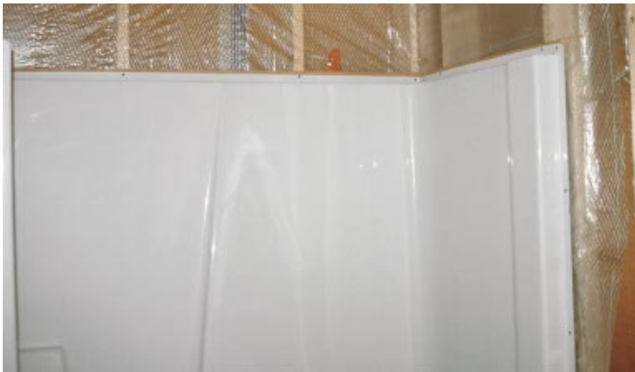
Figure 4. When a tub/shower unit is located on an exterior wall, the poly air barrier is installed before the tub goes in. To create a tight air barrier, the poly needs to be taped to the bottom plate of the wall.
