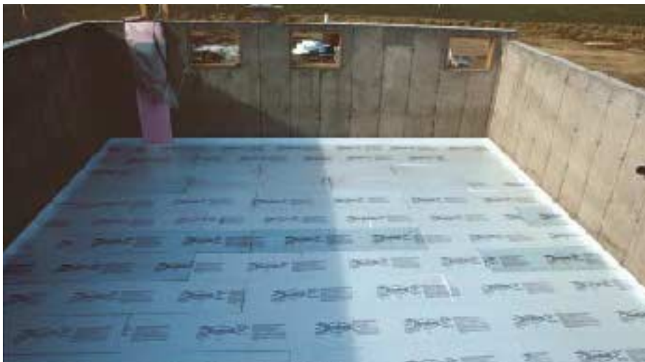
Figure 1. Installing 1 inch of rigid foam insulation under the basement slab keeps the slab warm enough to prevent moisture from condensing on it. The perimeter insulation between the slab and the colder concrete wall provides a thermal break. The cast-in-place pressure-treated window frames will receive low-e argon-filled windows.
