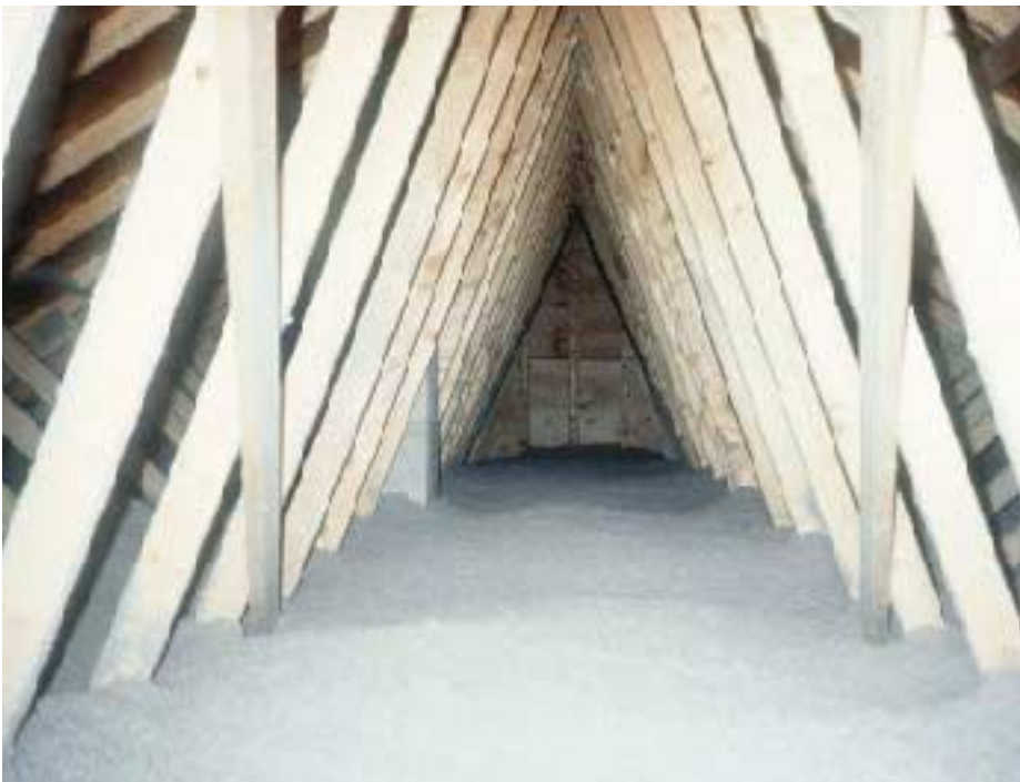
Figure 9. Cellulose insulation effectively fills all of the spaces around the bottom chords of roof trusses. Because cellulose is cheap, it can be piled on deep.
