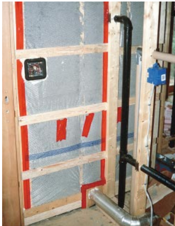
Figure 7. Where this dryer vent penetrates the exterior wall (at bottom of photo), a plywood block provides a surface for taping the poly air barrier. This house has horizontal wall strapping, so there was no need to recess the plywood block between the studs. Note that where the partition meets the exterior wall, the penetrations for the plumbing vent and electrical cable are sealed with urethane foam. The photo also shows an Enviroseal airtight electrical box.
