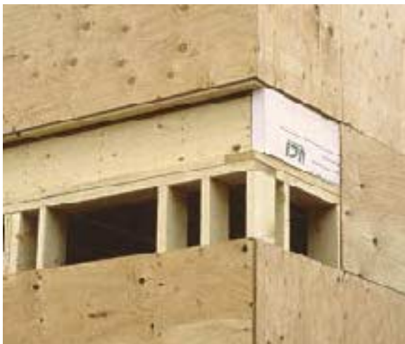
Figure 2. Recessing the band joist 2 inches provides room for exterior rigid foam insulation. To provide an air barrier, the foam is carefully caulked in place with Tremco acoustical sealant.
