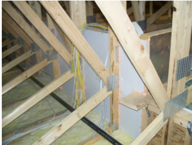
Image depicts a properly sealed air barrier at an attic knee wall.
