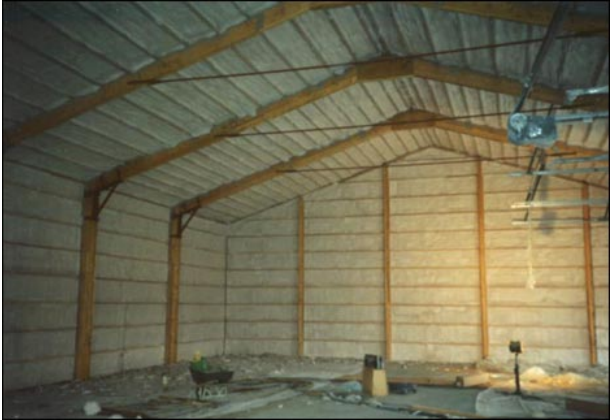
Commercial roof and wall – complete indoor climate control.
