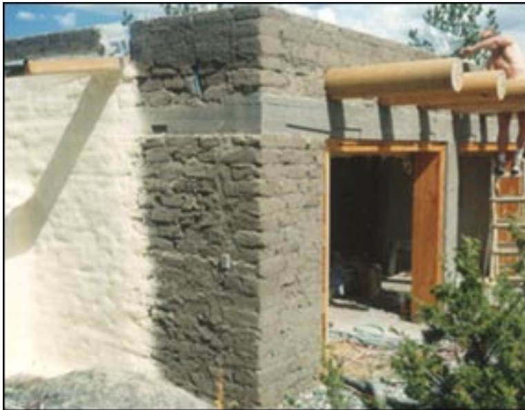
Closed cell spray polyurethane as air/moisture barrier, thermal insulation and stucco base over adobe.
