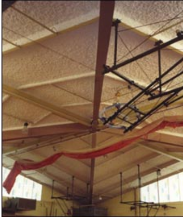
Junior High Gymnasium Bozeman, MT Accoustical thermal barrier finish applied direct to spray foam under roof deck.
