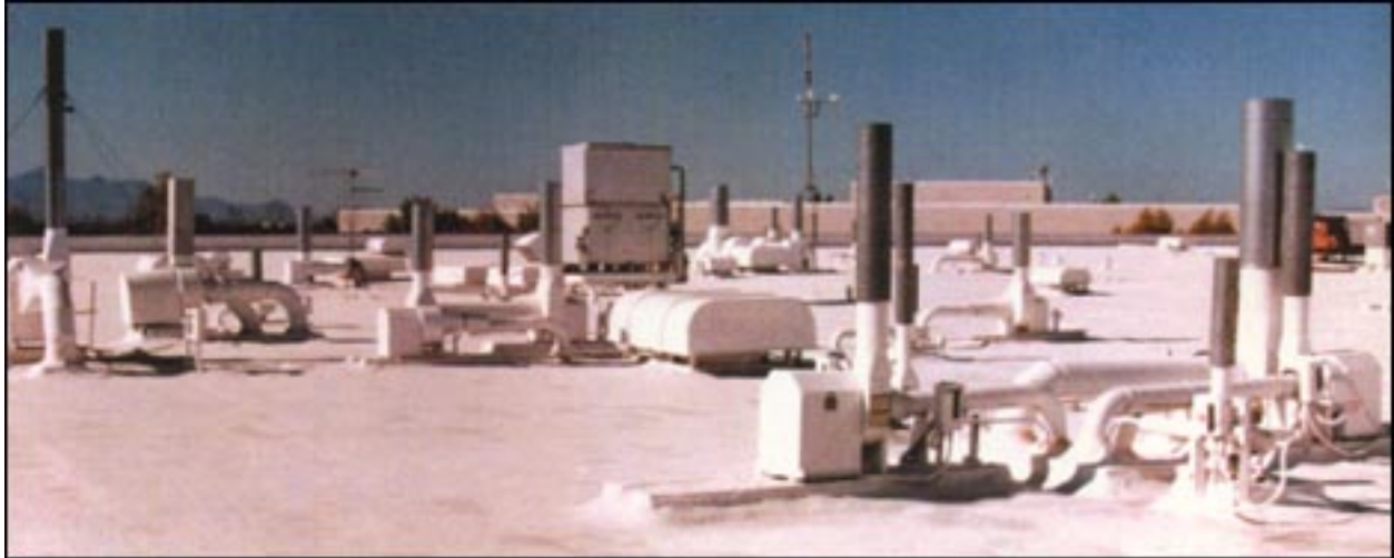
IBM – Courtesy SPFA ...with spray in place closed cell polyurethane foam and coatings.
