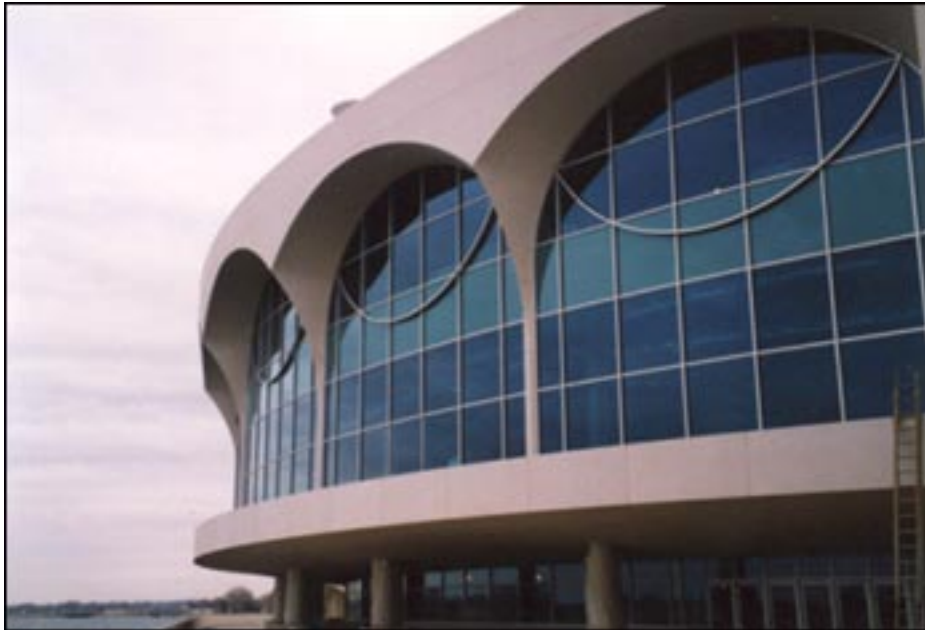
Monona Terrace Convention Center – Madison, WI Complex pre cast arch shapes require thoughtful attention to thermal, air and moisture impacts.
