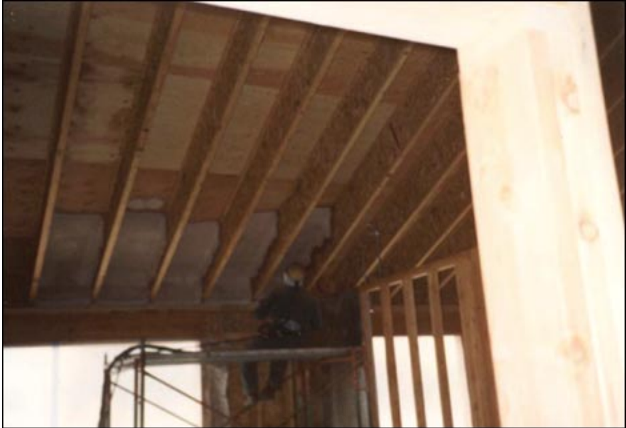
Boulder School, Boulder Montana 54,000 sq. feet of unvented cathedral roof installed in rafter lengths up to 48 ft. Application direct to underside of cathedral roof deck.
