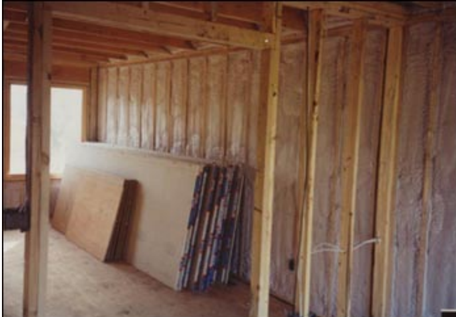
A wall ready for interior finish – no thin air/vapor retarder to sustain damage or be poorly installed.
