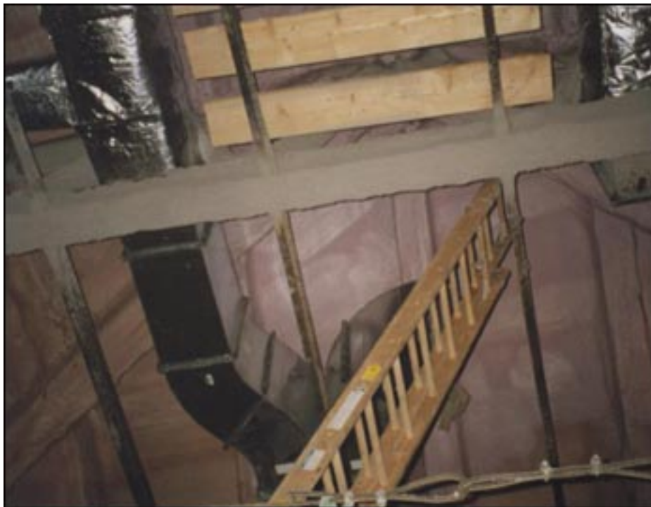
Harvard Law School Library Reconstruction Application up to cast in place concrete roof deck.
