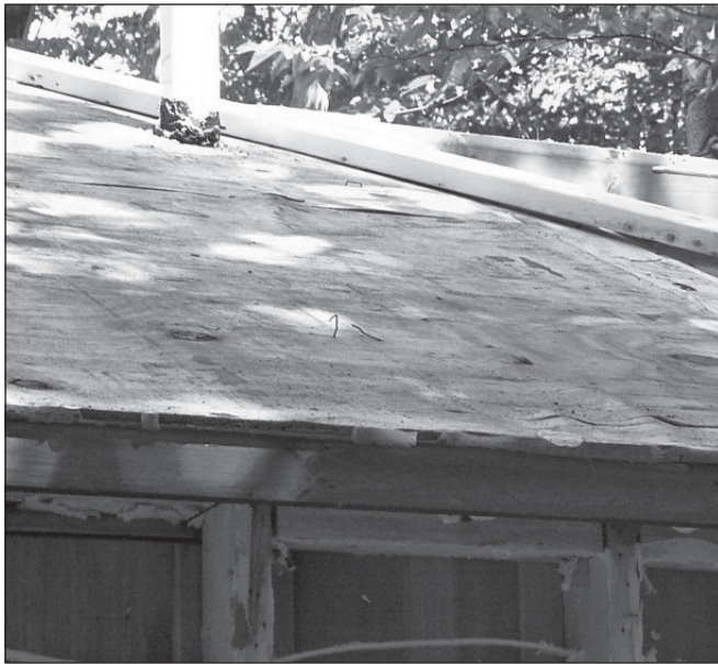
Figure 2. The cathedral ceiling of the Moffitt house became so saturated with moisture that the plywood roof sheathing showed signs of delamination and warping.
