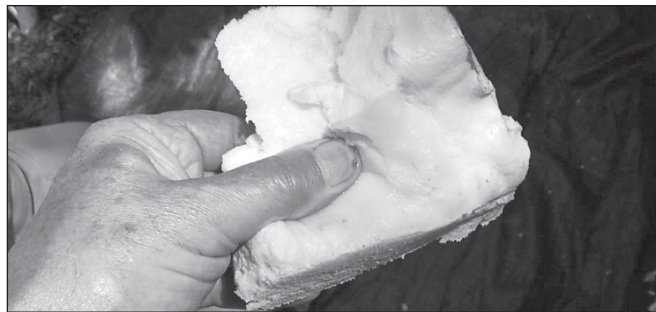
Figure 1. Icynene insulation is an open-cell foam that allows water vapor to pass through it by diffusion. At the Moffitt house, the walls were so wet that water could be squeezed out of the sponge-like Icynene.
