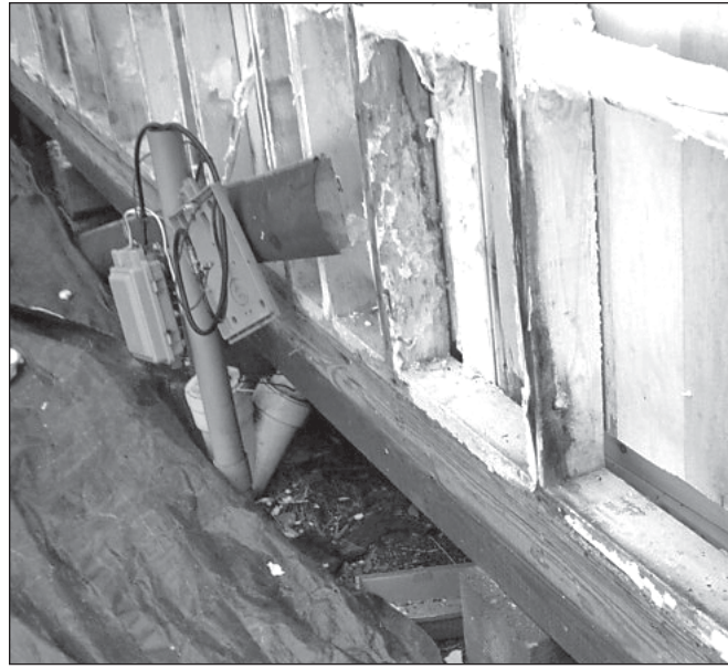
Figure 3. The stud bays of the Moffitt house were opened up from the exterior in order to remove the wet Icynene insulation. Many of the studs were black with mold.
