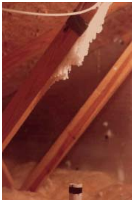
Figure 3. Moist interior air leaking through a hole in the ceiling can produce moldy sheathing or frost on a roof truss. This photo by the author shows results from the Attic Performance Project.
