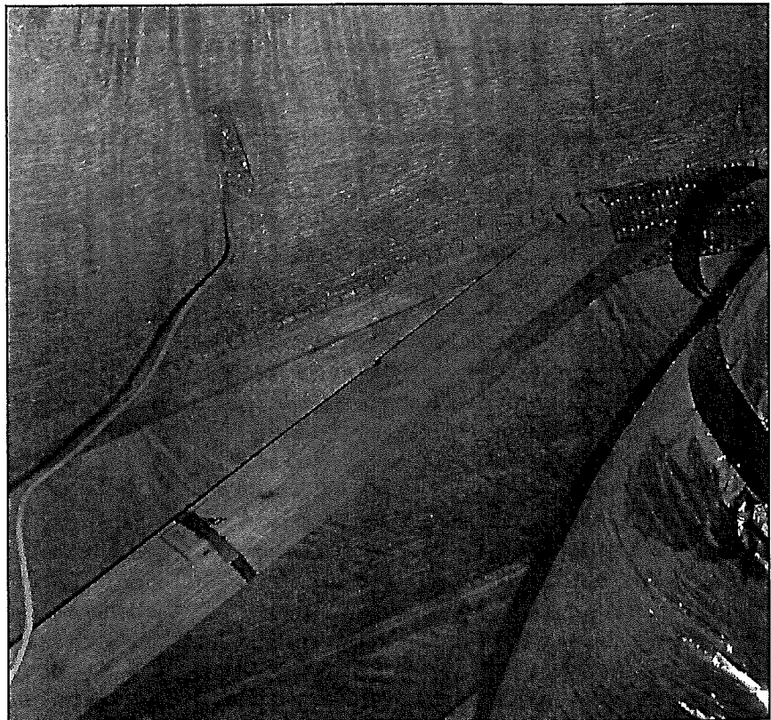
Figure 2. Air-permeable insulation, like this netted cellulose, should not be used to cathedralize an attic in a cold climate. The photo shows one of the roof assemblies in Phoenix, Arizona, studied by Armin Rudd; a HOBO temperature / relative humidity sensor is visible on one of the truss chords.
